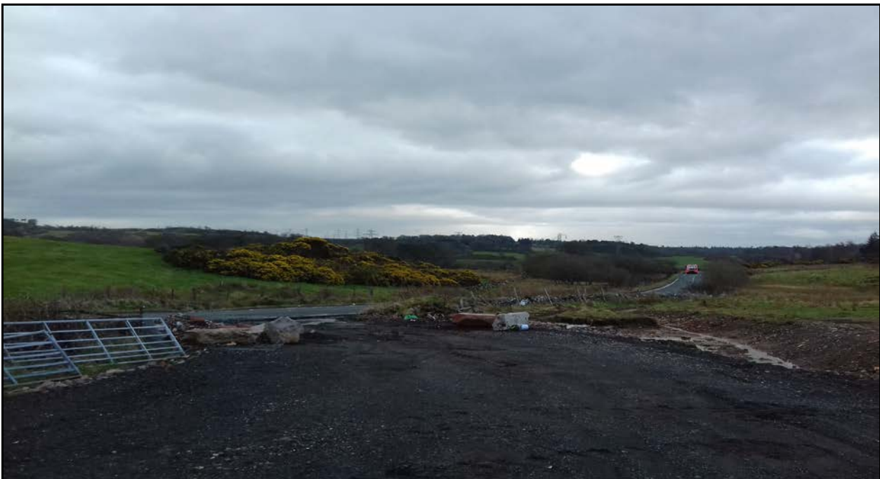
View of the access point as currently constructed looking towards Port Glasgow Road
